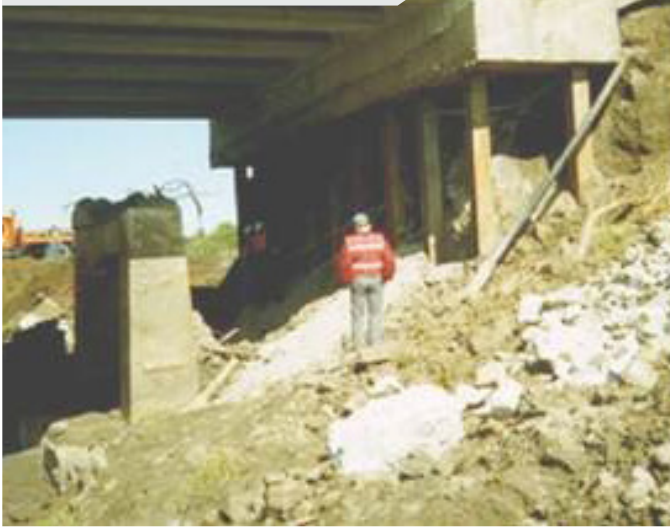
Photo 3: Bridge Abutment Damage Due to Scour
