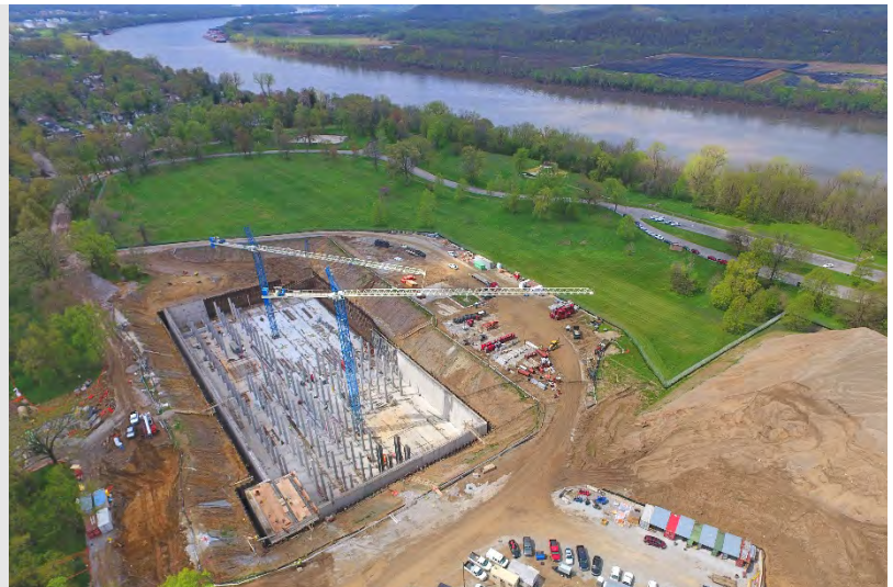
Figure 32. Construction of a 20 million-gallon CSO storage tank along the Ohio River. Once completed, the tank will be hidden underground and used to protect the river by preventing combined sewer overflows.
