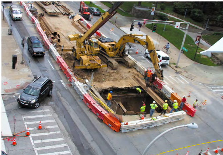
Figure 30. Failures of large-diameter sewers create huge impacts. This cave-in closed several lanes of a busy intersection. Communities need to be able to fund preventive maintenance projects to address aging infrastructure.
