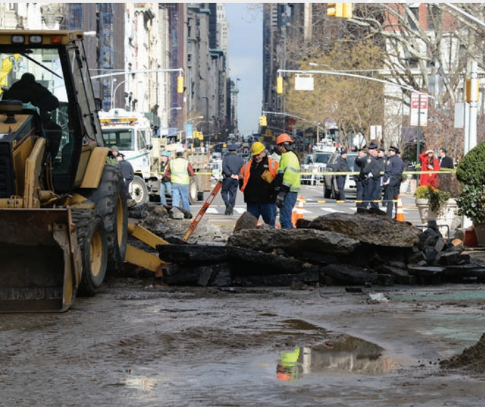
Crews worked to pump water from the track bed and restore N, Q and R train service after a 36-inch water main broke at 23rd Street and Broadway on February 1, 2013.
