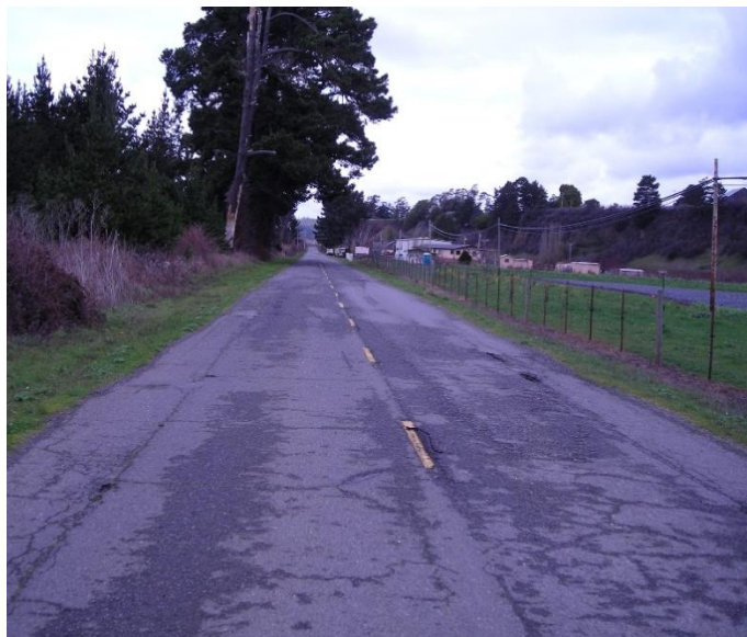
Figure 3. Existing asphalt concrete deteriorating on Eel River Drive near Fortuna, CA.
