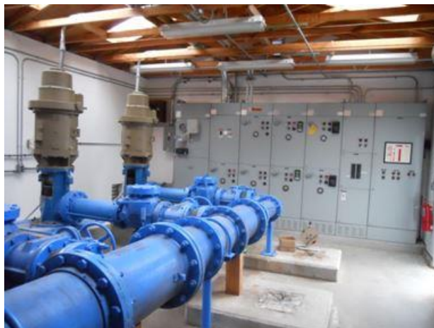
Figure 4. City of Fortuna Relocation of the Electrical Panels at the Corrosion Control Facility to above the estimated flood elevation for a 100-year storm event.
